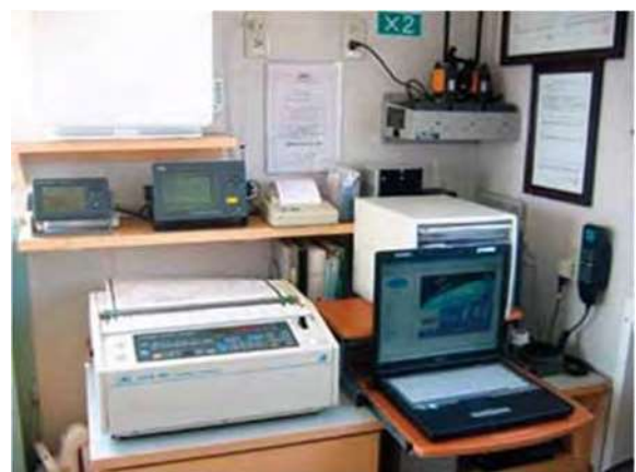
無線区画－2／Radio equipment area-2
