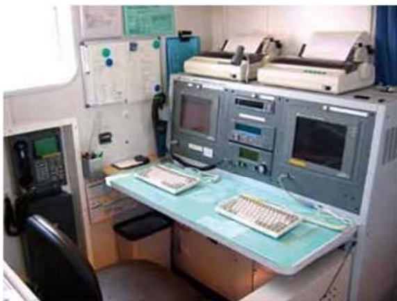
無線区画－1／Radio equipment area-1
